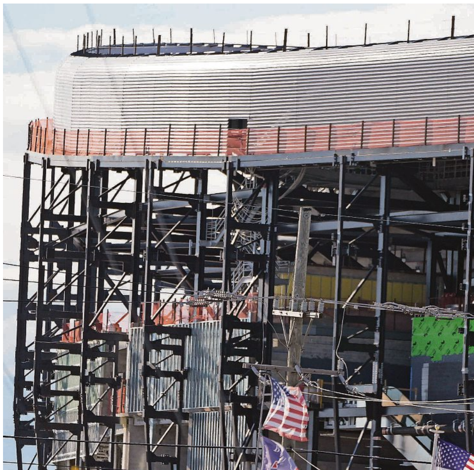
Construction progress at the new Highmark Stadium in Orchard Park is shown Sept. 7. TINA MACINTYRE-YEE/ROCHESTER (NEW YORK) DEMOCRAT AND CHRONICLE
